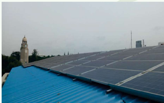
Figure 2: RTPV Installation at BESCOM premises
