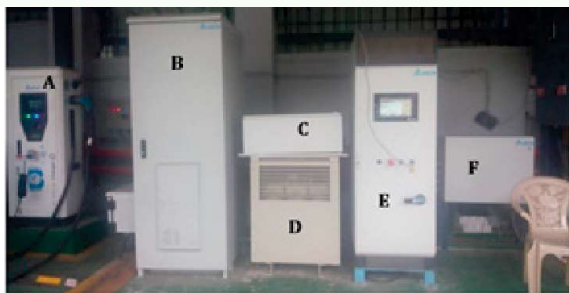
(A: Bharat DC 001 charger, B: lithium-ion battery bank, C: MPPT block, D: transformer, E: PCS, and F: distribution box)
